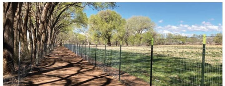
..... Photos show the new trail and fencing installed around the East Field at the Del Norte Open Space property.
